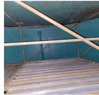
Inside of Baby Creek chemical tank #2; new spray on liner with scaffold for further spark testing.
