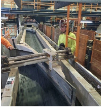
Sludge Bypassing Conveyor P-11/12 Plow
