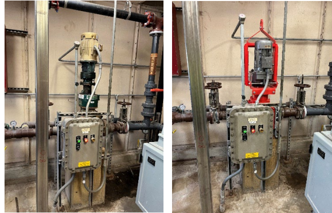
The old grinder faced similar clogging issues experienced with the belt filter presses and has been replaced with a more modern model
