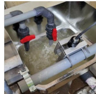
Total Suspended Solids (TSS) sensor at Primary Effluent (PE) sampling location
