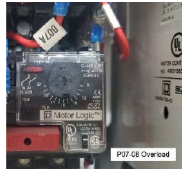
Conveyor P-7/8 Overheated
