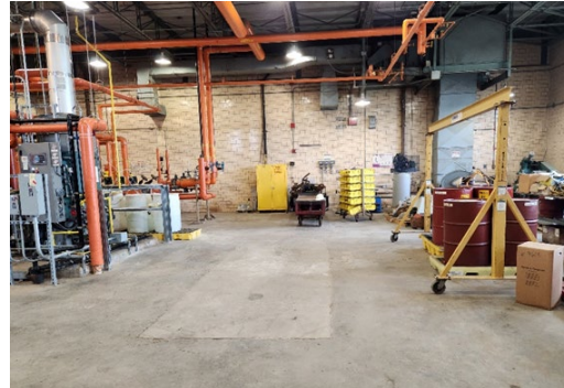
WWP boiler area
