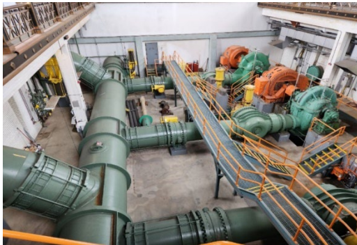
WWP high lift pump area
