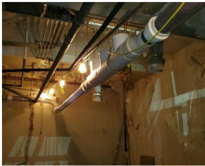
New Ferric Chloride Piping At PS-1 Pre-work Inspection
