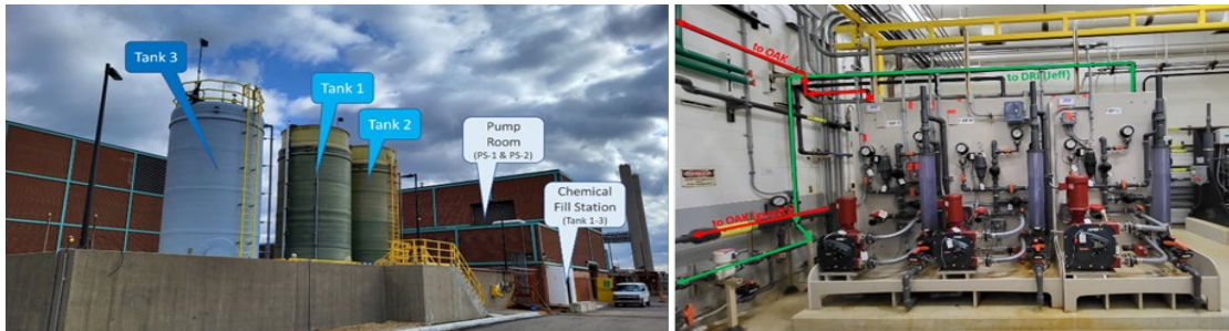
Ferric Chloride system at Pump Station 2 servicing both pump stations (left) Pump skid feeding to Pump Station 1 in the Pump Room (right)
