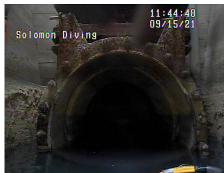
Missing flap gate as found during initial inspection
