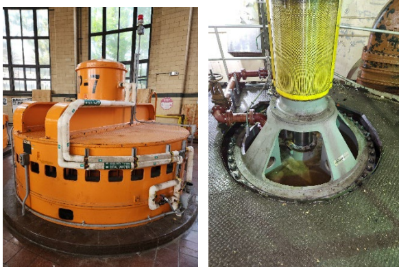
MLP #7 immediately after being released back to operations upon the initial start-up testing
