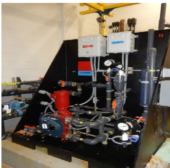
PS-2 Ferric Chloride Pump Skid
