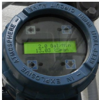
PS-2 Ferric Chloride Flow Meter
