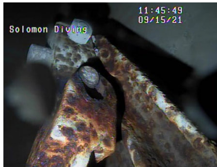
Condition of gate hinge as found during initial inspection
