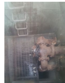
I-Valve Vault at North Service Center
