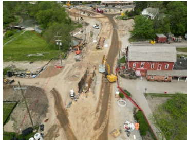
WTM installation near the Yates Cider Mill
