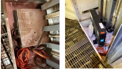
Old (left photo) and new (right photo) UPS installation.
