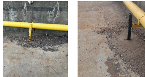
One of the old, corroded pipe supports, and the replaced support prior to painting. The new supports will be painted yellow to match the natural gas piping as shown in the photos
