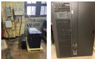
PS1 (left) and PS2 (right) New UPS
