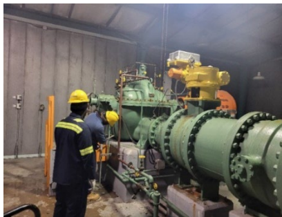
Marcus Jackson and Veyon Bentley doing preventive maintenance at West Service Center
