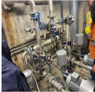
Left is the crew recalibrating valves at in-system storage device (ISD) #5 Lovett Street
