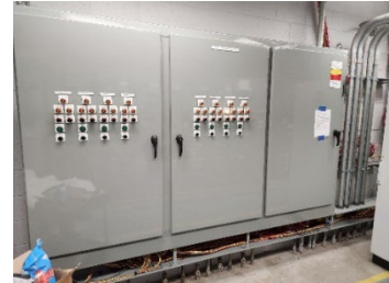
New Baby Creek CSO Screens Control Panel
