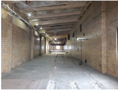
New switchgear room after removal of the abandoned equipment and initial cleaning
