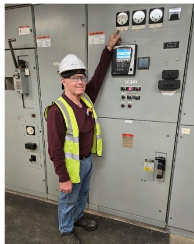
Power Management Electrician George Barnette pointing to the obsolete High Temperature Relay
