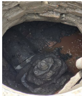
Valve located underground at Stage 3 – Michigan and Rosa Parks
