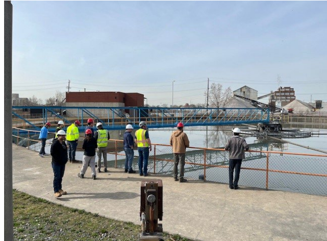
Members observe a clarifier during a tour of the Water Resource Recovery Facility on the April 10 th with the WWBP Work Group
