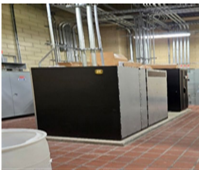
New breaker equipment at Springwells Water Treatment Plant
