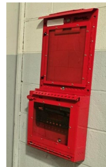
LOTO box mounted in Complex II Dewatering
