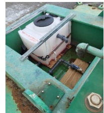
Pilot shaft mixer fluid pilot test
