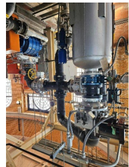
The new priming system at Conner Creek SPS
