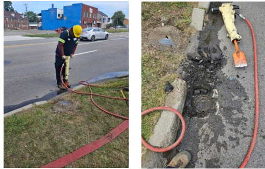
Field Service Technician Caleb Ogunnupe obtaining access to valve associated to Water Resource Recovery Facility field testing
