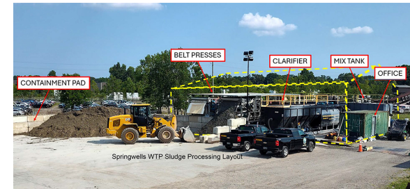
Basins Sludge Processing Facility
