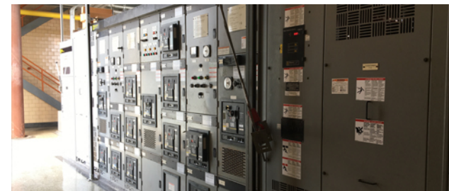
Service Building Electrical Substation
