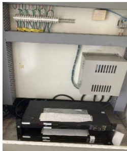
New power transfer switches at WRRF De-Chlorination
