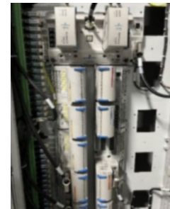
Control Cabinet Testing during St. Aubin/Leib Factory Acceptance Test shown (photo blurred intentionally)
