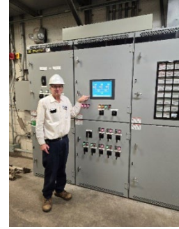
Team Leader Ray Zdonkievicz showing the new PLC display. Ray was responsible for coordinating the electric plant testing
