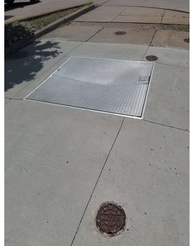
Unable to unlock meter pit door
