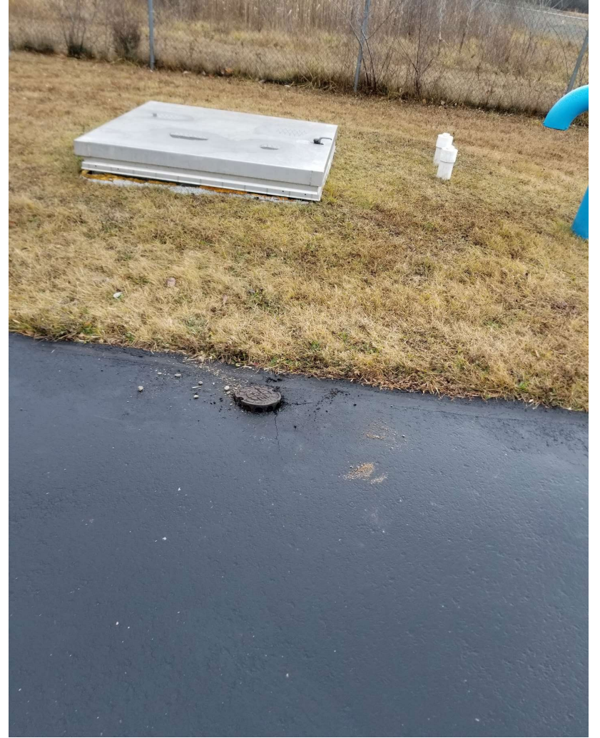
Not Accessible, Excessive Debris on Valve
