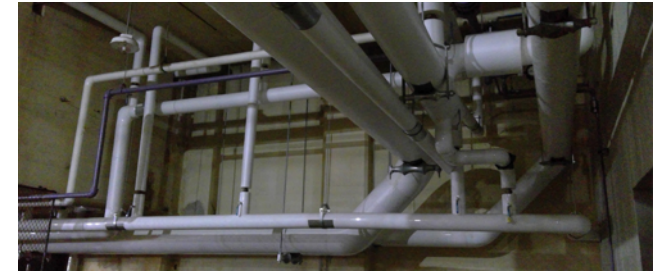
Condensate Return, and Compressed Air Piping
