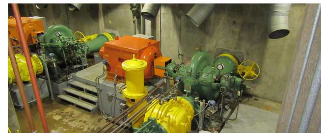
Adams Road Pumping Station
