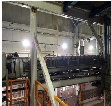
New lights at conveyor K
