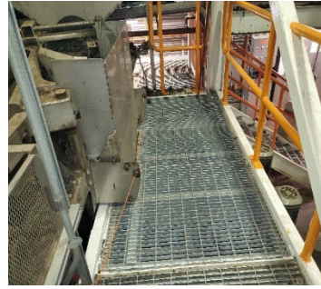
Extended Maintenance Platform at P9 and P10
