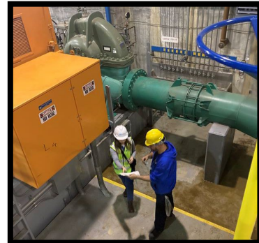
Figure 2: EAMG’s Ashley Zimelman and Field Services Ian Sizemore at Franklin Pump Station
