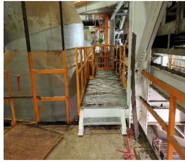
Maintenance Platform at conveyor K and L
