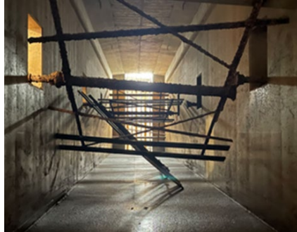
Existing flocculation equipment Sedimentation Basin #4
