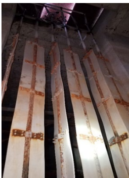
Existing inlet controls
