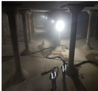
Interior of Springwells WTP Reservoir #1
