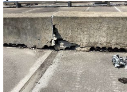
Existing Concrete Enclosure Failure at HS
