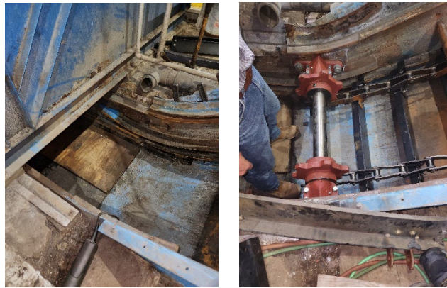
The inflection point of Grit Flight 1 where the flights start moving up to move grit to another conveyor. These pictures are before and after the sprocket installation.
