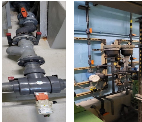
Leib Screening and Disinfection Facility (SDF) chemical room
