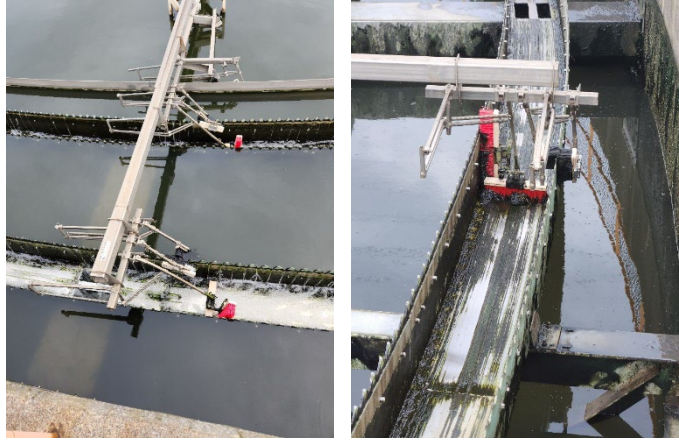
Rehabilitated brush riggings installed on a secondary clarifier
