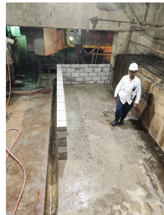
Operations Team Leader Joseph Rowland, looking at the newly constructed containment wall in the Pump Station 1 basement
