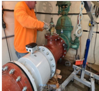
Meter Pit SE-09 14 Mile Road and Lasher
