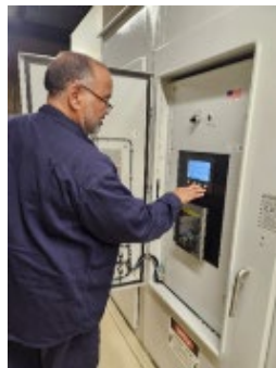
Dave West at Imlay Station looking at the soft starter for our Line/Reservoir #5 Motor to find out why it is tripping off. He is checking the settings in the starter to make sure it does not have any issues there.
