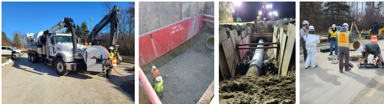
GLWA Maintenance and Repair team assisting with cleaning the 48-inch water main, additional pipe segment installation and replacement, and the HDR pipeline inspection team
