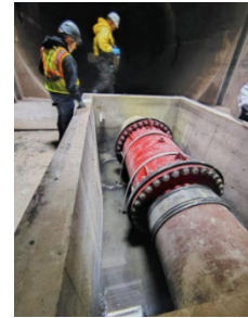
Pinch valve at Oakwood Pump Station
