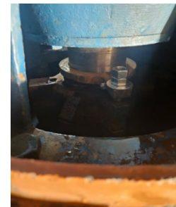
Pump No. 9 at Freud Pump Station
