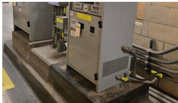
Southwest's battery charging system
