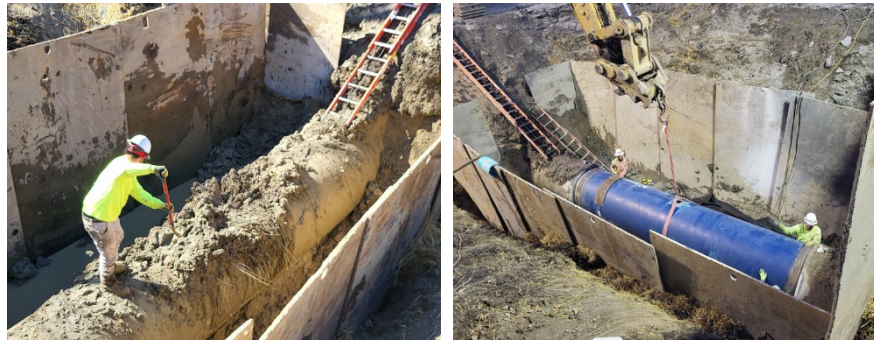
48-inch water main break and repair pipe
