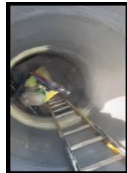
The long periods between wet weather affords the team the time to perform this inspection activity as shown in the image above
