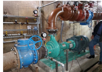
Newly installed SFP No.2
