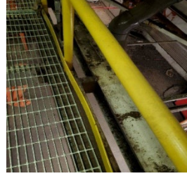
Extra support for maintenance platform
