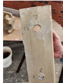
Additional clip found that showed signs of failure; currently being replaced
