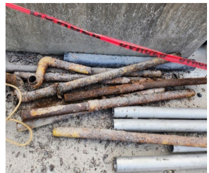
Failed gas line
