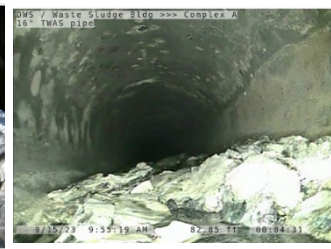
Lining from Pickle Liquor Tank 1
