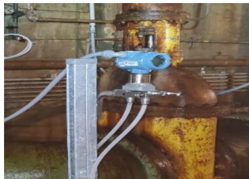
NEWTP new loss of head meter (Typical 1 of 88)
