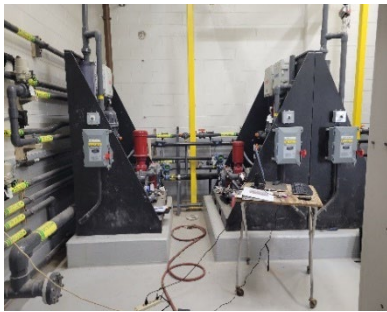
PS-2 Ferric Chloride Pump Skids
