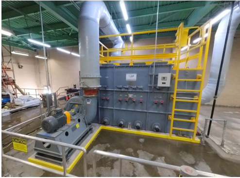
SWWTP new scrubber
