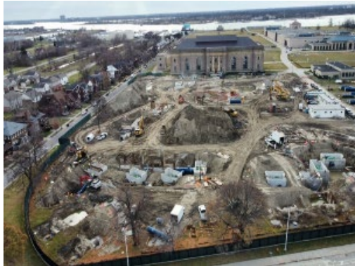
Aerial view of WWP High Lift Pumping Station mid-construction of eastern portion
