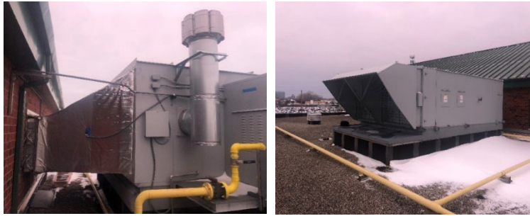
The newly installed makeup air unit-2 is shown in the left and right
