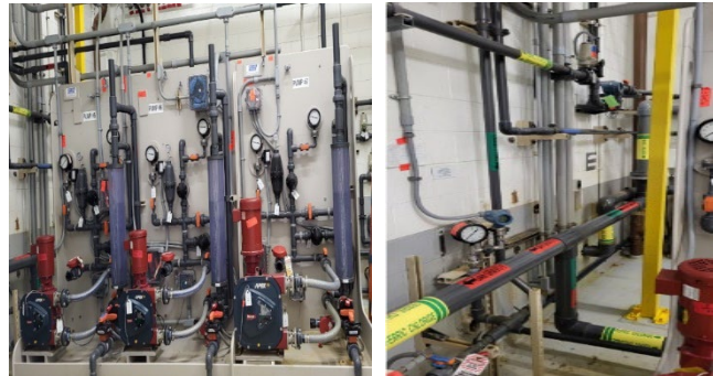
Ferric Pump Room at Pump Station 2
