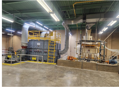
SWWTP old and new scrubber side by side
