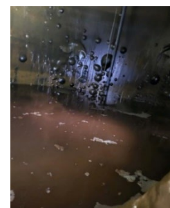
The discolor of NaOCl shows chemical is behind the liner
