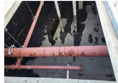
Basin 2, looking down through the equipment lowering hatch at Hubbell-Southfield.
