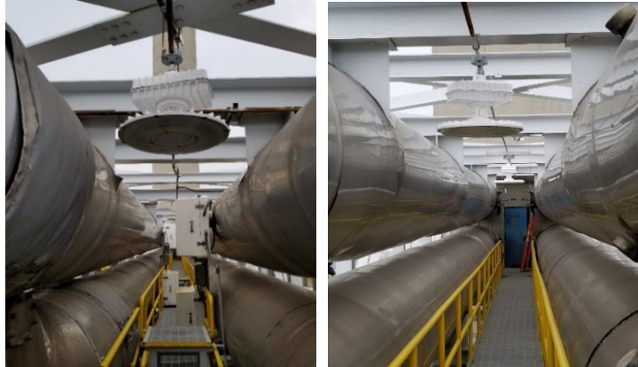
New light fixtures installed on the catwalks to the tall stacks at WRRF
