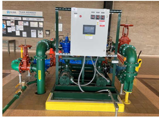
SWWTP raw water screen booster pumps
