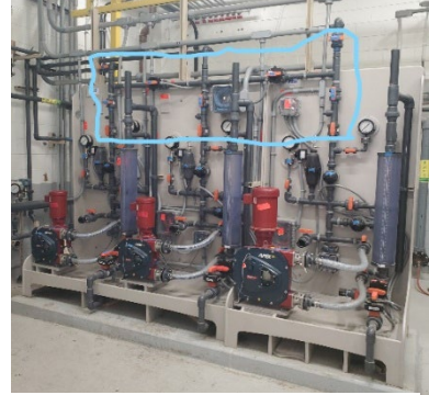
Unreachable Valves at Ferric Chloride Pump Skids
