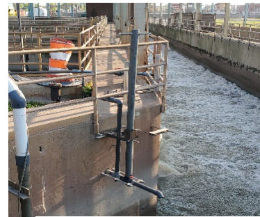
PS-2 Discharge Channel Ferric Chloride Feed
