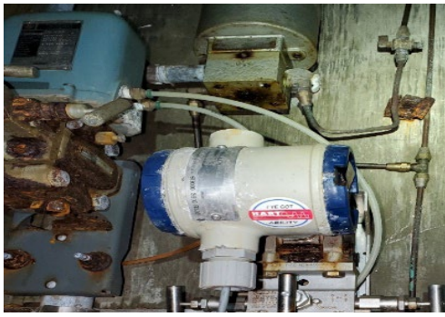
NEWTP old loss of head meter
