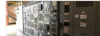
Service Building Electrical Substation
