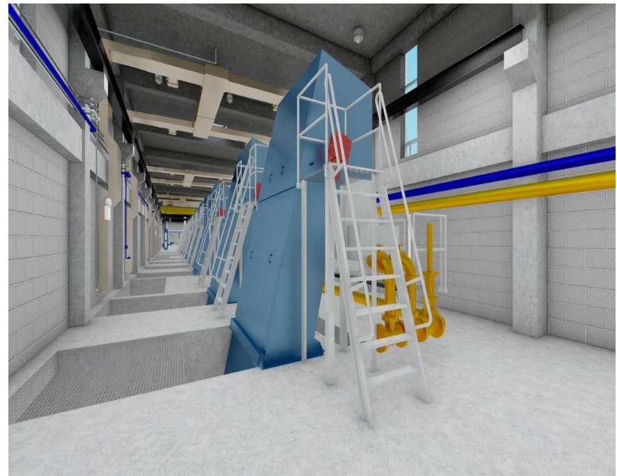
\frac{1}{4} " Bar screens (10 total)
