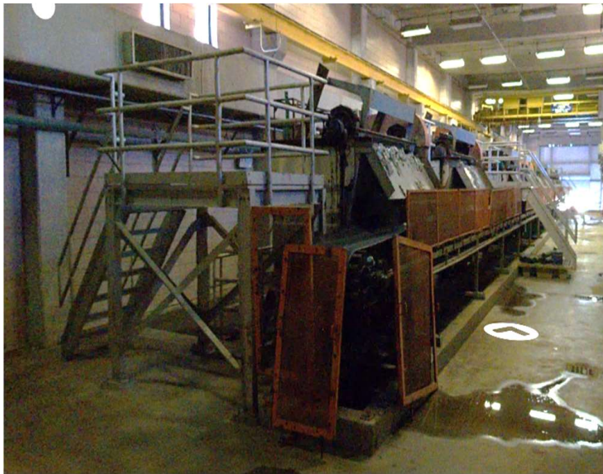
\frac{3}{4} " Bar screens (8 total)
