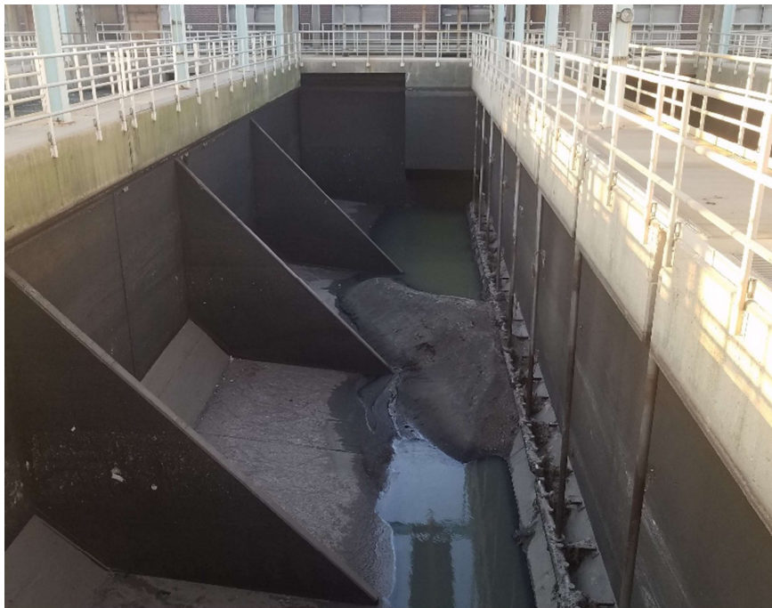
Aerated channels with weirs (8 total)
