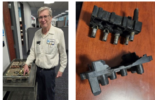
Left: Team Leader Ray Zdonkiewicz indicating the location of the faulted UPS connector. Right: connector removed from the UPS above.
