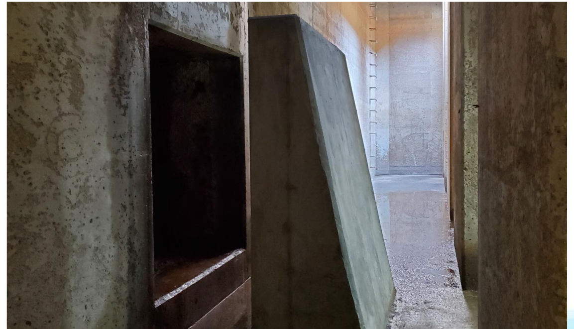
Flocculator Basin Inlet Baffle
