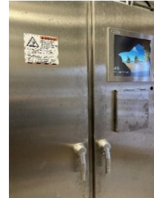
The new network cabinet (left) and new controls cabinet (right) are shown above
