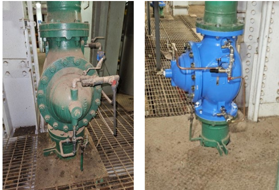
Old PRV and new replacement PRV
