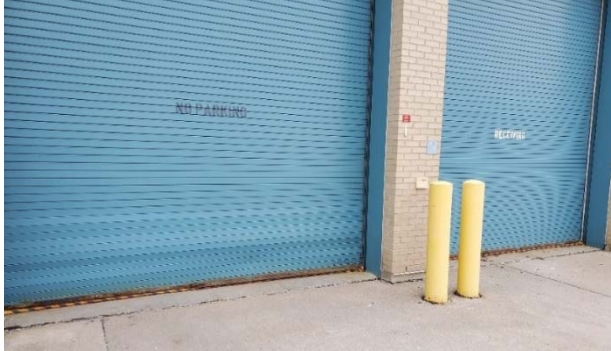
Bottom Slats and Safety Deeteriorated
