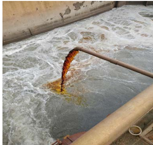
Ferric Chloride feed into PS#2 discharge
