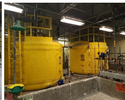
Phosphoric Acid Bulk Tanks
