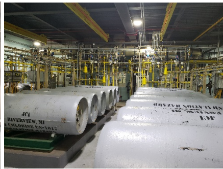
Chlorine Storage Room
