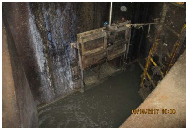
Deteriorated regulator chamber
