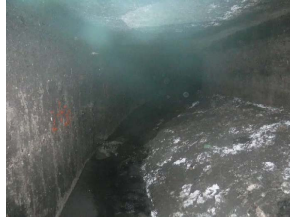
Accumulated Debris in the conduit
