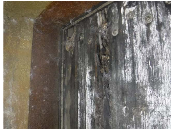
Deteriorated Backwater Gate
