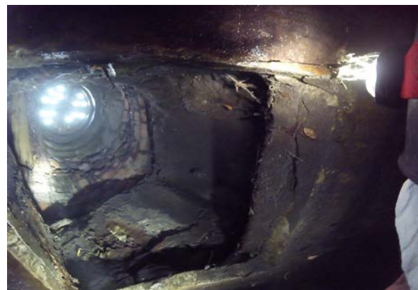
Poor manhole condition
