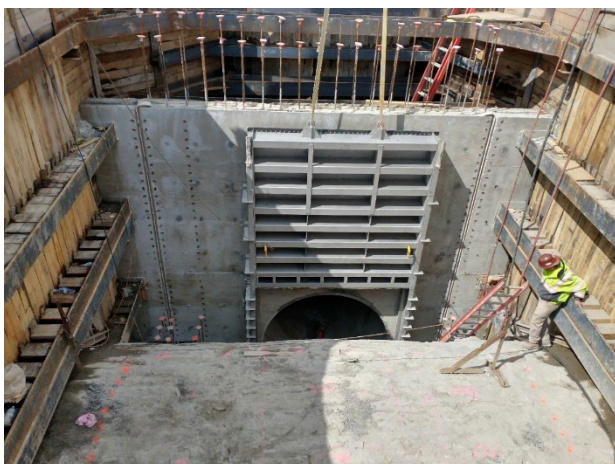
DRI gate installed during test and flow directed to NIEA through connection
