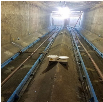
Underground Grit Channel
