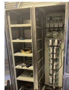
New Network Cabinet (left, devices not installed) and New Controls Cabinet
