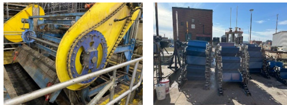
The new drive shaft, sprockets and chain on Bar Rack #3 and the buckets and chain are being prepared for Grit Collector #3
