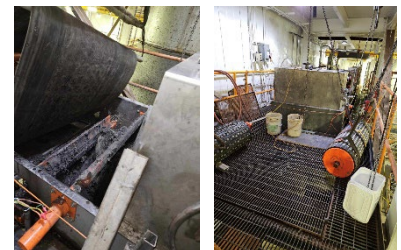
J-conveyor head pulley is removed, and the new head pulley staged for installation as shown in the left and right photos above
