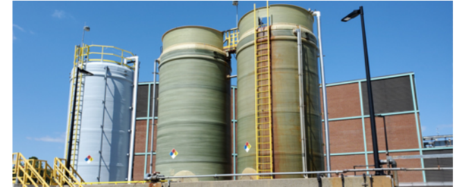
Rehabilitation of Various Sampling Sites and PS#2 Ferric Chloride System at WRRF
