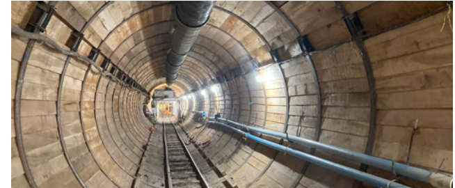
Detroit River Interceptor (DRI) Evaluation and Rehabilitation
