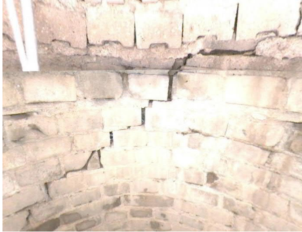
Figure 8. Sample Manhole Defect from a Manhole in the Five High Priority Neighborhoods
