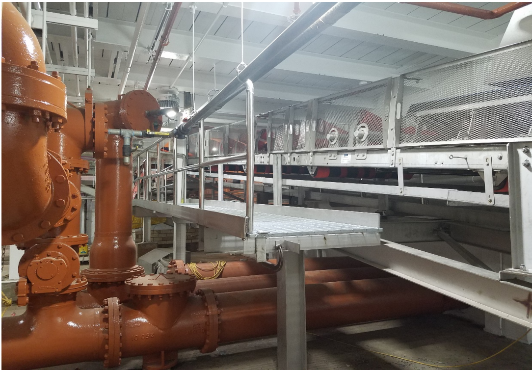
New belt conveyor ‘E’, structural stainless steel, and re-coated Complex II basement walls, ceiling, and process piping
