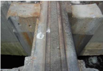
Piece of movable dam at DRO-2
