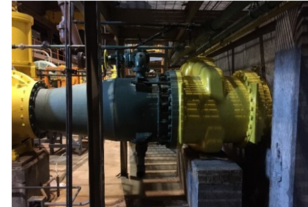
Isolation gate valves
