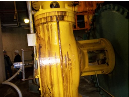
Oil hydraulic valve actuators leaking oil
