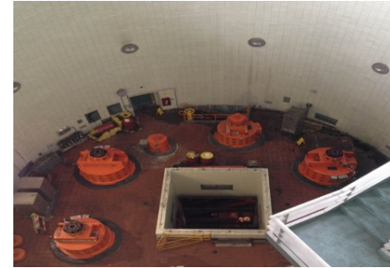
Low Lift Pumping Plant at Northeast WTP
