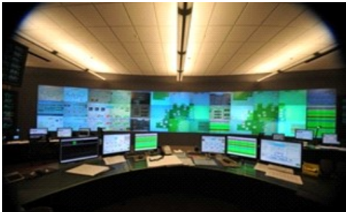
A system control room
