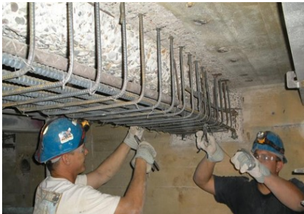
Lake Huron WTP Electrical Tunnel
