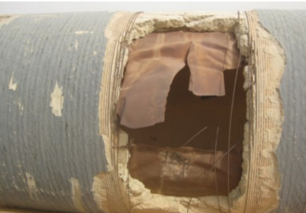
Example of a failed water main
