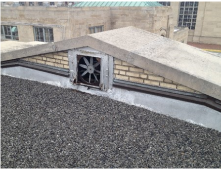
Roof in need of repair
