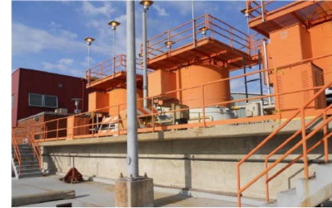
Intermediate Lift Pump Station N.2
