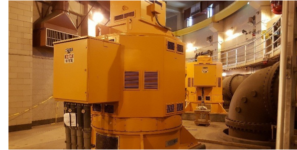
Main Raw Sewage Pumps at Pump Station 2
