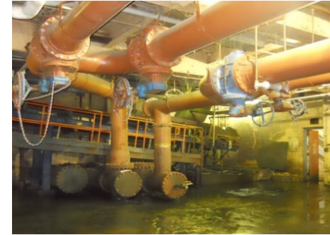
Sludge Feed Pumps
