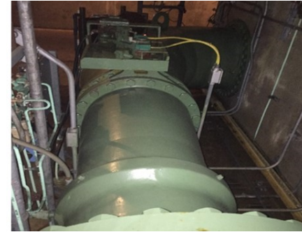
Raw Water Flow Meter
