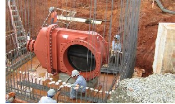
A large valve for a transmission pipe
