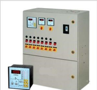
Energy management to reduce energy costs
