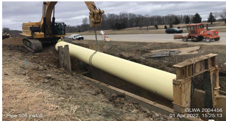
Pipe installation for the 14 Mile Loop project, which eliminated a single feed for 250,000 people in Oakland County
