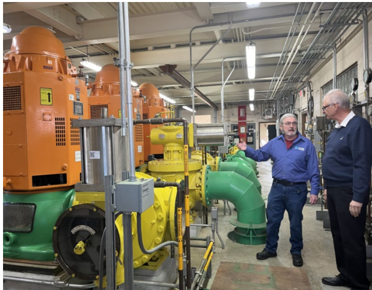
West Chicago Booster Station
