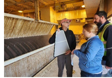
Charles Wrigley, Wixom Operator, explains how to clean the disc filter system (similar to the future equipment for CIP-216008) to Laboratory Manager Andrea Busch, Wastewater Operating Services Laboratory Manager, and Chad Cogar, Wastewater Operating Services Maintenance Manager
