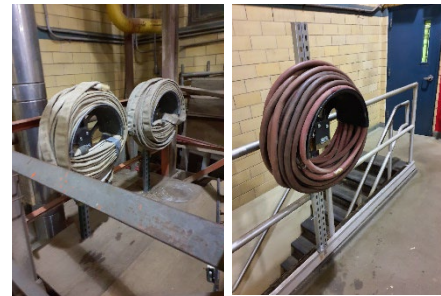
Some of the new hose reels that were installed around the boiler room for easy access and restorage of hoses
