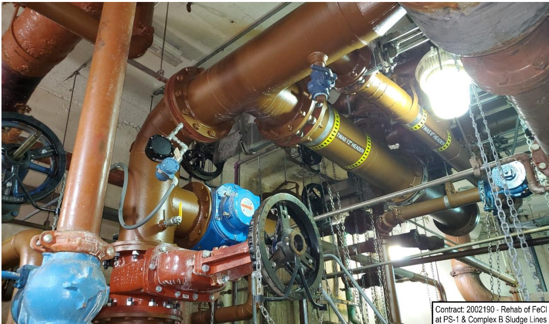
Complex B Sludge Piping Reconfigured for Cleaning
