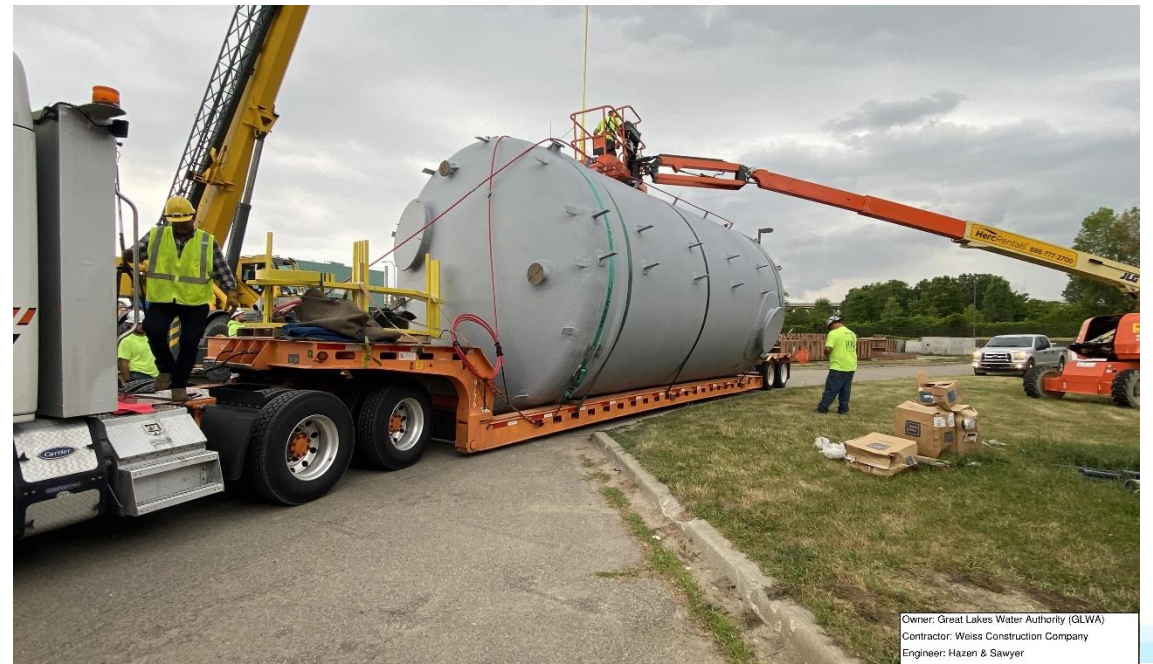
July 2022 Ferric Chloride Tank Delivery
