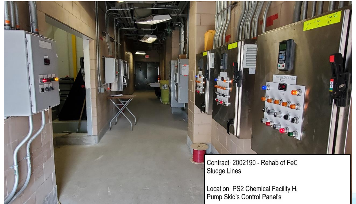
May 2023 Ferric Chloride Pump VFDs Installed and Being Tested
