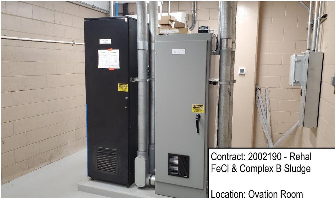
May 2023 Ovation Control System Panels Installed and Being Tested
