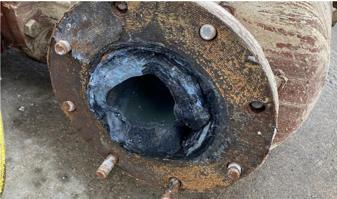
January 2022 Vivianite Mineral Buildup In Removed Complex B Piping
