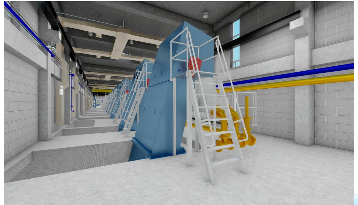
1/4" Primary Bar Screens (10 Total)
