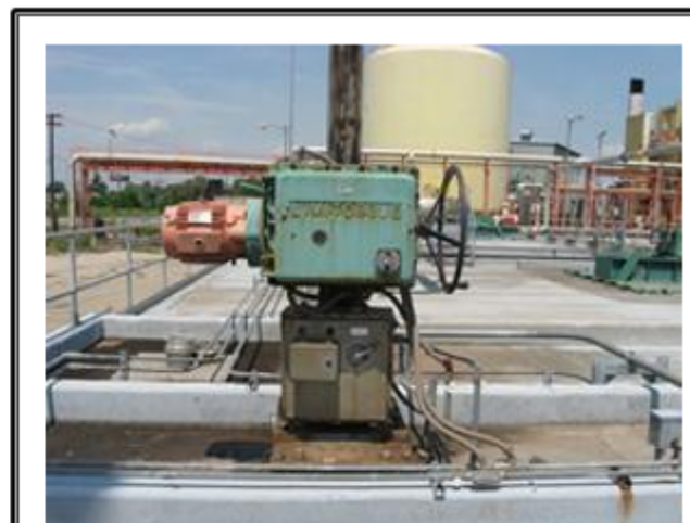
Equipment for aeration system
