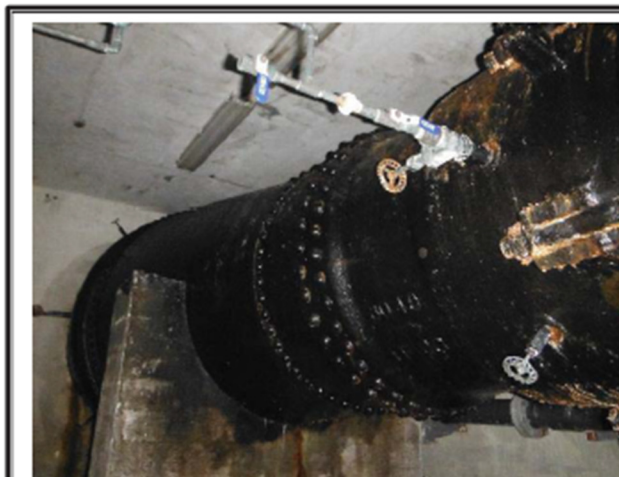
Water production flow metering device
