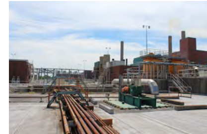
Aeration Basin 1 and ILP's 1 and 2
