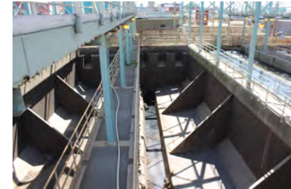
Pump Station 2, Grit channels
