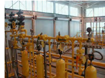
Chlorination Building, Inside
