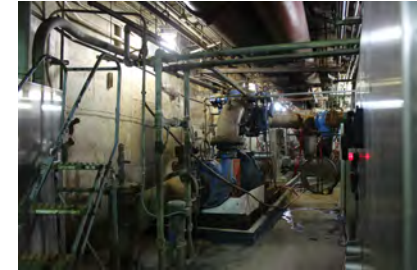
Sludge Feed pump in Complex A
