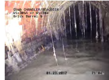
Woodward Sewer System
