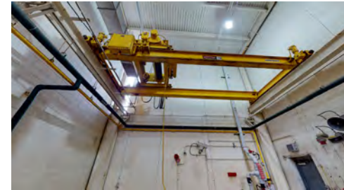
Coroded building crane from failed HVAC system
