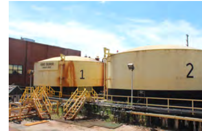
Ferric Chloride Storage and Containment Area
