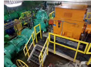
Inside Joy Road Pumping Station
