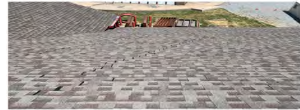
• The previous installation on roof area 2 also failed to follow the required "step-down" installation method. As seen in the picture above, the shingle seams fall >4" from each other. This is a very common mistake found on
