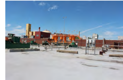
Aeration Basin 4, and ILP's 3, 4, and 7
