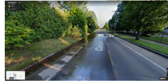
Photo of the berm leaking into Clairpointe
