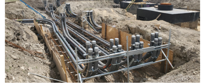
Low-Lift and High-Lift Pumping Station Improvements
