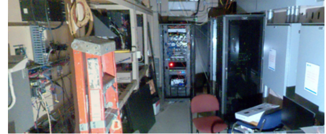
Lake Huron Water Treatment Plant, Filter Instrumentation and Raw Water Flow Metering Improvements
