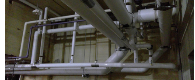
Condensate Return, and Compressed Air Piping
