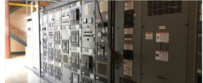
Service Building Electrical Substation
