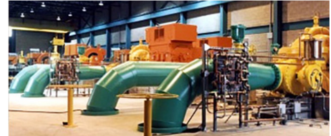
Franklin Pumping Station
