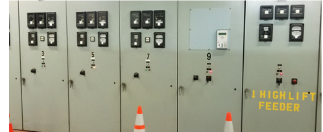
Lake Huron Water Treatment Plant
