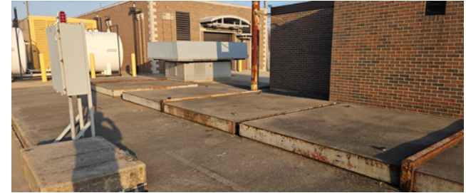
Schoolcraft Pumping Station
