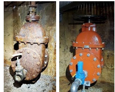
Existing (pictured left) and new (pictured right) drain valves. Main valve is 10-inch, secondary valve is 2-inch.
