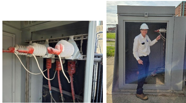
Team Leader Ray Zdonkievicz pointing out the incorrect wiring and a close-up photo of the incorrect wiring used
