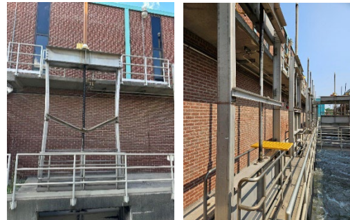
SG-9B with a bent frame and frame support and SG-9b after repairs pictured in the left and right photos
