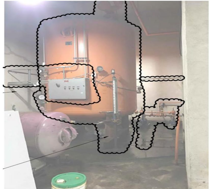
Old Oil-Pneumatic Tank
