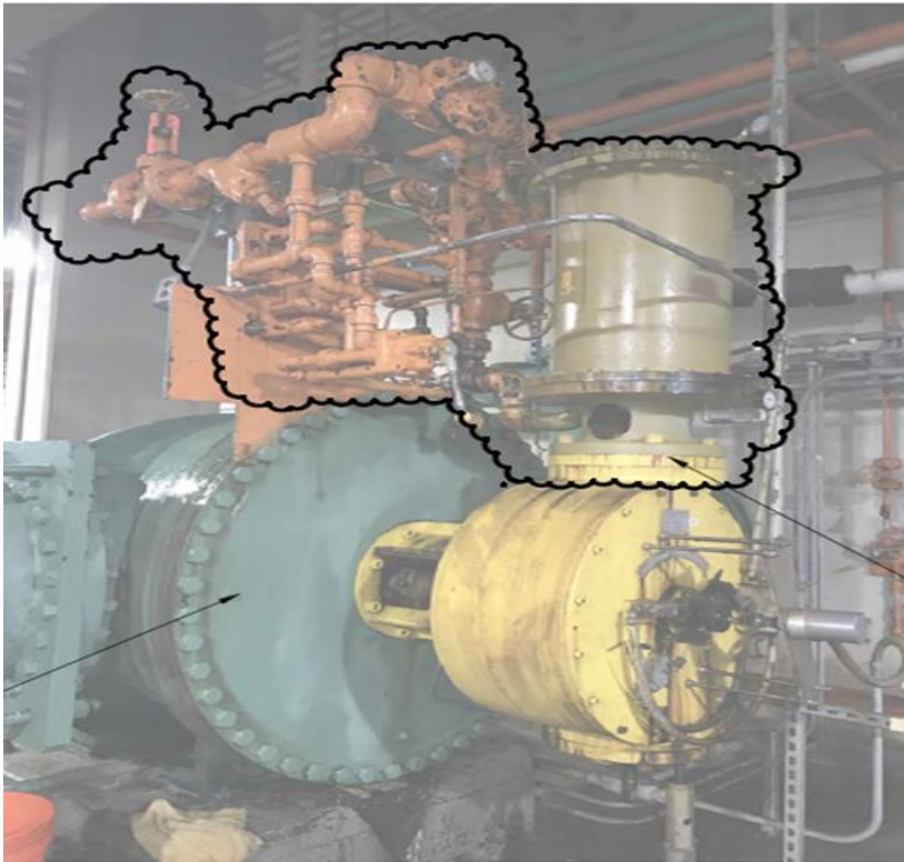
Old Oil Hydraulic Actuator (typical)
