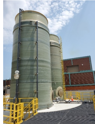
Ferric Chloride tanks and associated pipes, electric and controls, platform and rails
