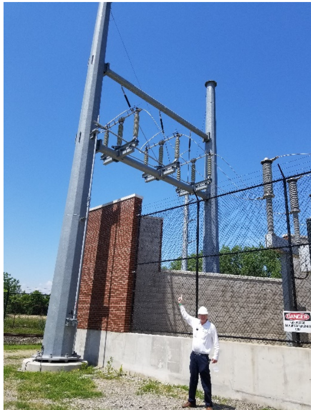
H-Frame with third 120,000V power source to the WRRF
