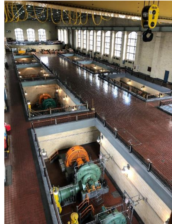
High Lift Pumping Pits
