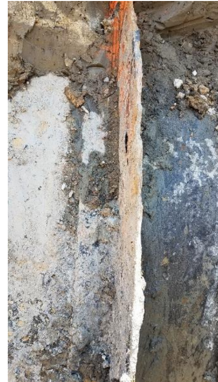
Corroded Flange on Main #5
