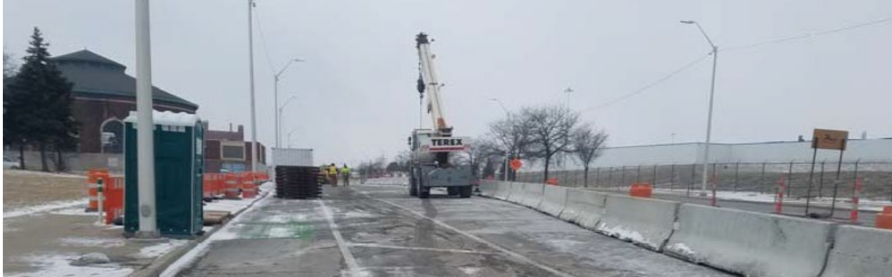
Barrier Installed at work zone east bound Jefferson at Connor for Access Shaft
