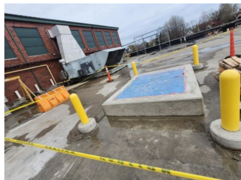
The newly installed FSP#2 Hatch at Conner Creek CSO
