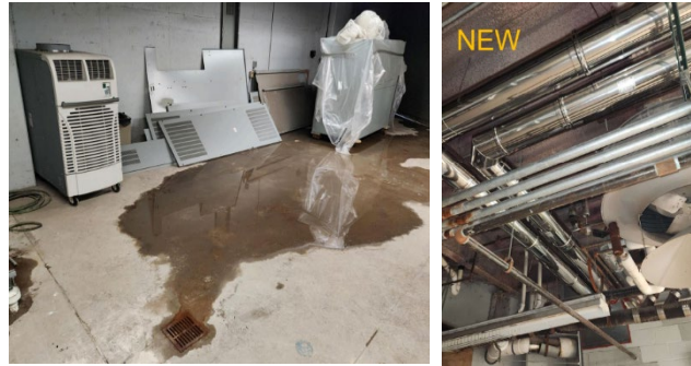
Left: Standing water from the leaking flue piping. Right: A section of the replaced pipe.
