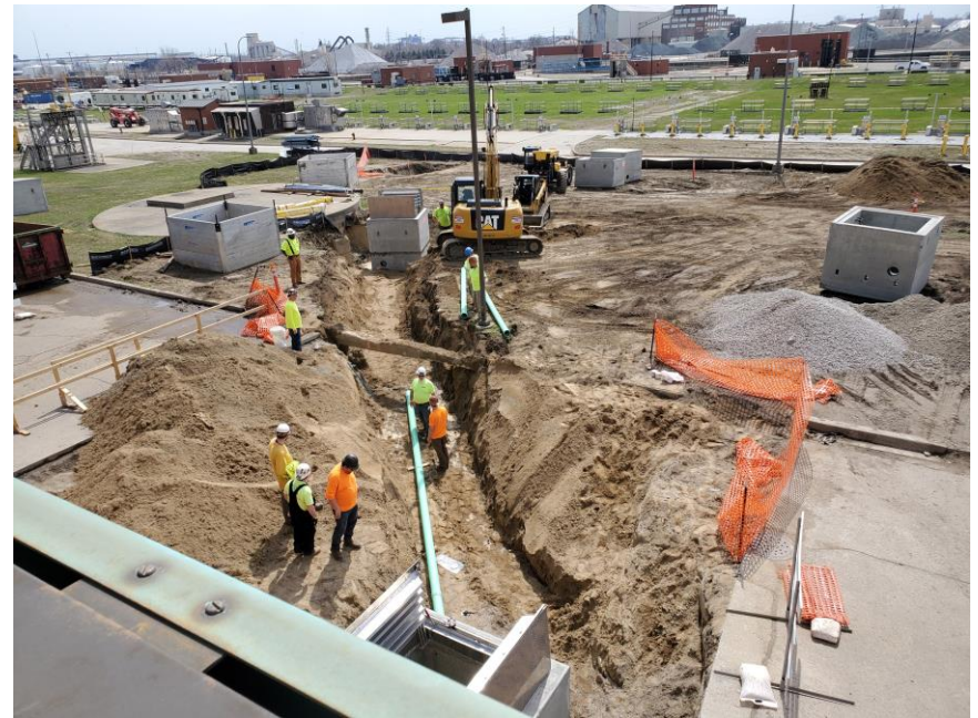
Installation of new pullboxes (PB-1 through PB-4) between PS-2 and pipe gallery completed Spring 2022
