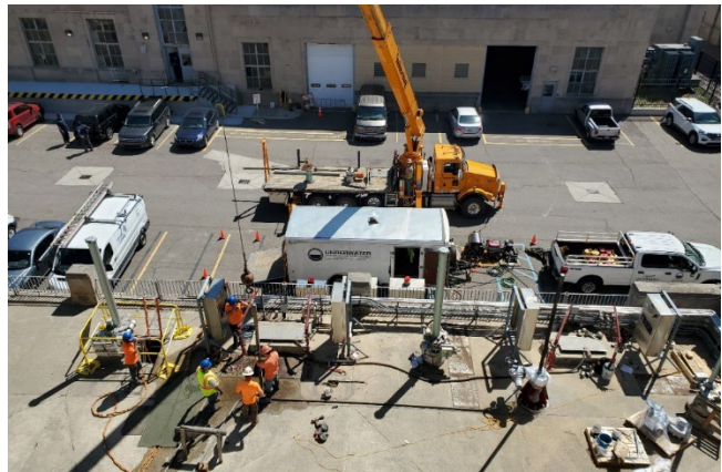
Overview of project site with one stem being installed (L) and one already in place (R)
