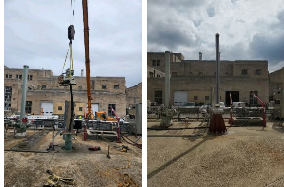
Left: Old stem during removal showing bend. Right: New stem and actuator
