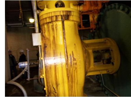
Oil hydraulic valve actuators leaking oil
