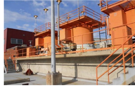
Intermediate Lift Pump Station N.2
