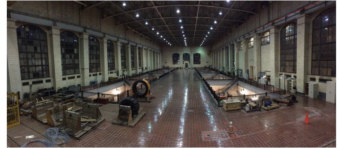
High Lift Station viewed from Low Lift Station operating floor showing high lift pump pits and windows to be replaced.
