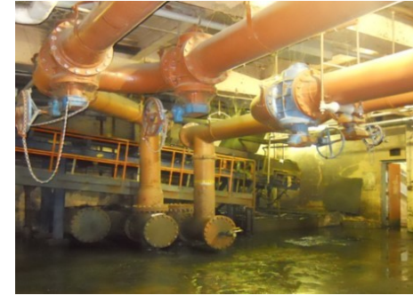
Sludge Feed Pumps
