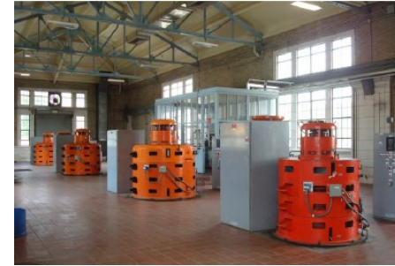
Sanitary pumps at Fairview Pumping Station
