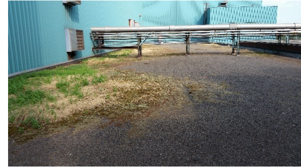
Photo of Complex – I Dewatering Roof at the WRRF. Complex – II Incinerator ($1.8M) and Complex – II Dewatering ($1.0 M) replacement are under consideration to be part of fire remediation project
