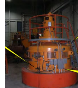
Pump at the Northeast Pumping Station
