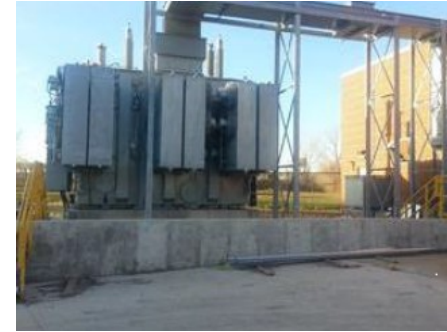
Electrical Duct Bank
