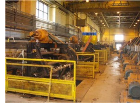
Rack and Grit
