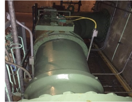
Raw Water Flow Meter
