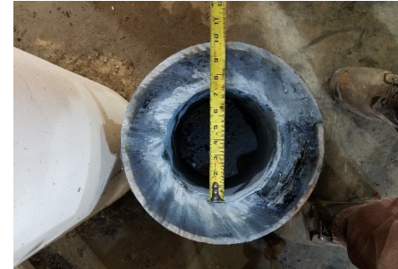
Complex B Sludge Lines clogged due to Struvite
