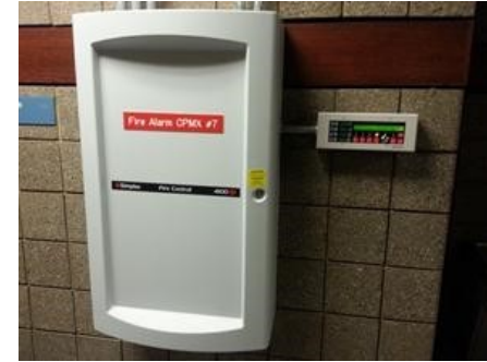
Fire alarm system
