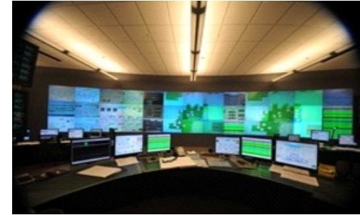
A system control room
