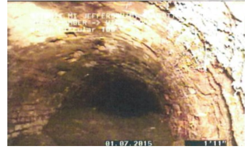
Sewer tap piping in B009 outfall (left) and sludge buildup and poor masonry in B007 outfall (right)
