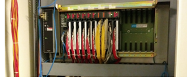
Control System Upgrade - St Aubin, Lieb and Mile
