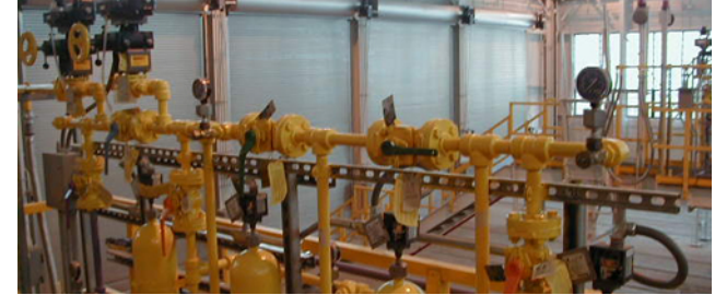
WRRF Conversion of Disinfection of all Flow to Sodium Hypochlorite and Sodium Bisulfite
