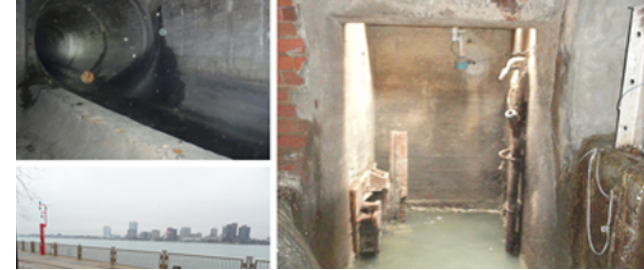
Sewer System Infrastructure Improvements and Pumping Stations
