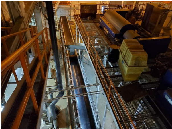
Newly installed replacement B-belt Conveyor (seen from third floor)
