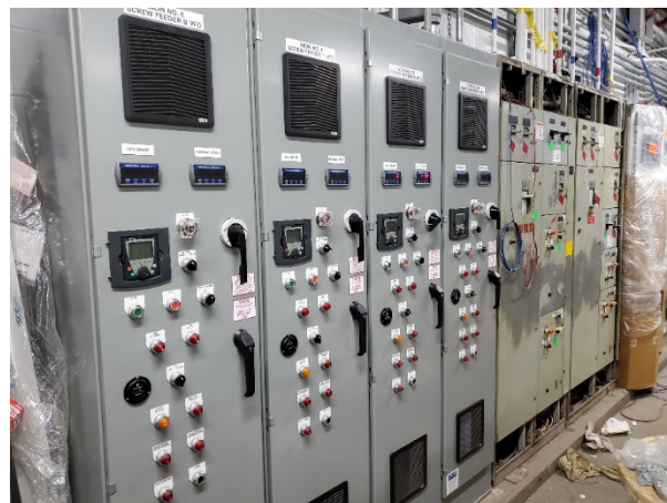
Newly installed and commissioned screw conveyor VFDs
